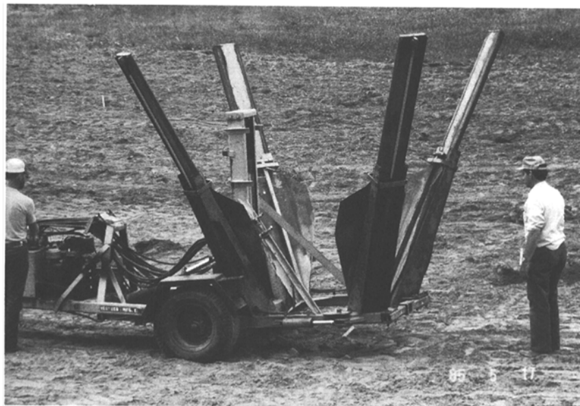
Fig. 2. Use of Vermeer tree spade to lift up a cone of soil at each vine site, to facilitate fitting the cone-shaped fiberglass barrier around each vine.
